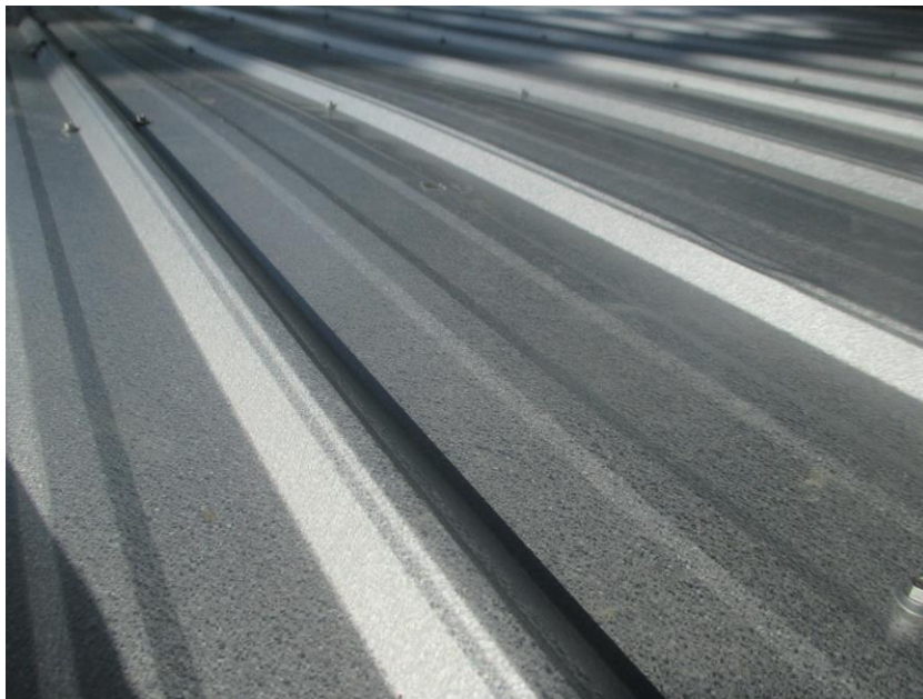
Specimen No. 2 After Testing
